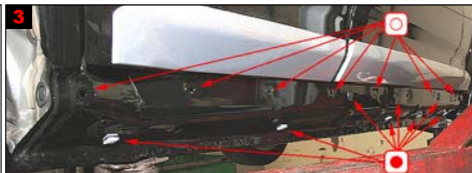
3 Panels: Remove cover plate. (Remove 5 screws and pul) Treat via existing and plugged holes.
